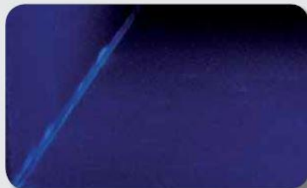
picture 18 detail of the residual dirt highlighted by the Wood lamp in the proximity of the corner of the P3ductal careplus duct
